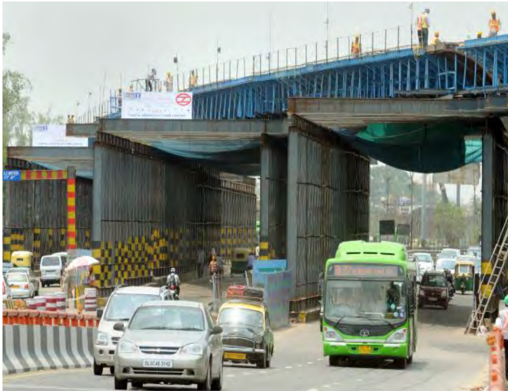
Construction underway in 2009 for the high speed railway line connecting New Delhi railway station with the international airport.
